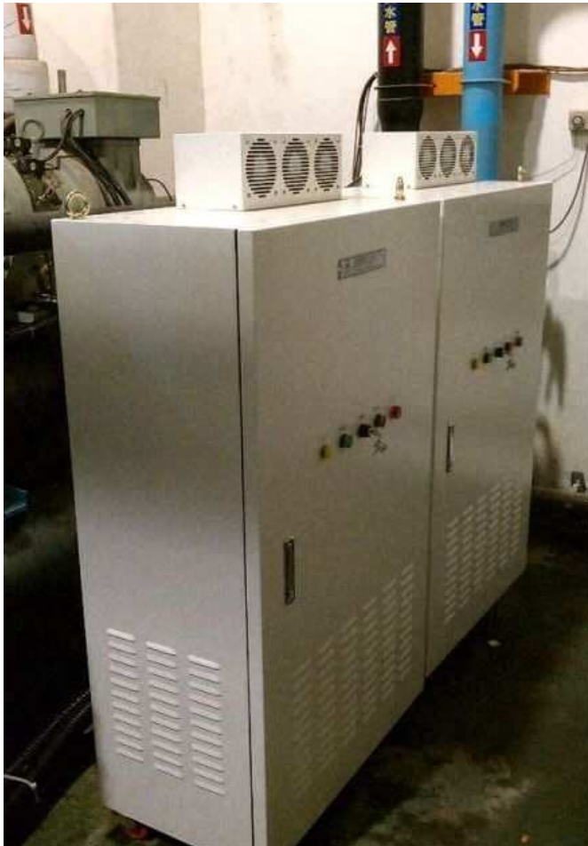
Energy saving for chiller
